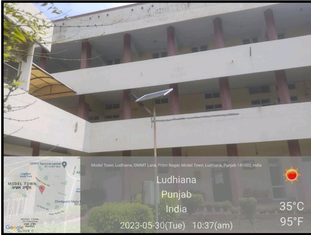
Solar lights installed in the campus
